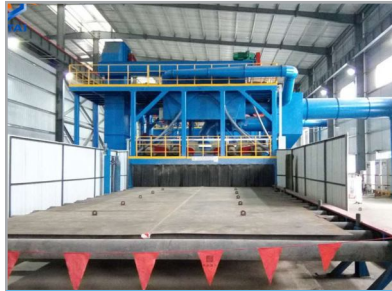
Shot Blasting And Painting Facility
